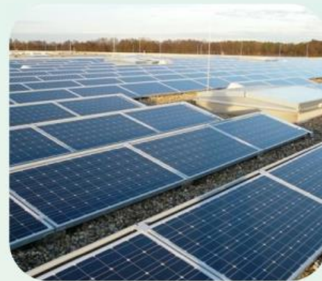
ROOF TOP PV LEIPZIG 5 MW
